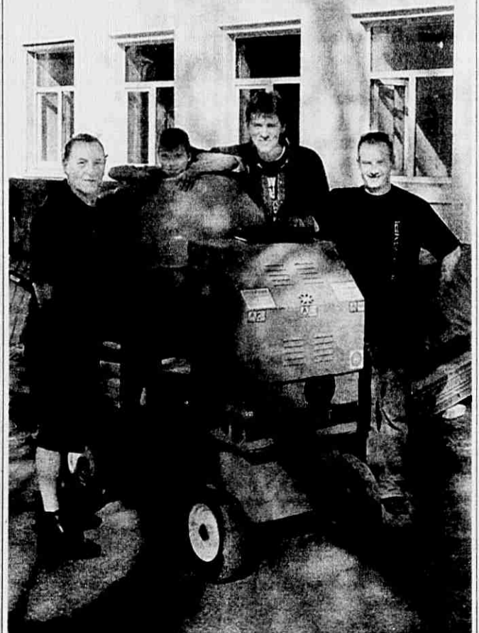
Tony O'Sullivan and Kevin Bannon from Dungarvan and Robert Reidy from Frreele about to start work with a mixer they have just unloaded from Ireland. Included is Ivana, a little helper from the orphanage.
