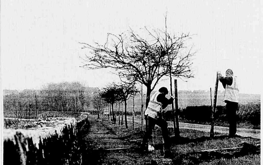
Pictured above Comeragh Landscaping planting a whole series of trees on what will be one of the most beautiful walks in Dungarvan. The line of new trees are planted along the path that meanders beside the Colligan Estuary stretching from the corner at The Mart right down to Ballineety Bridge and includes trees such as Ash, Birch and Lime. Well done to the council for identifying such a beautiful natural resource for the town and enhancing it for the enjoyment of the public.
