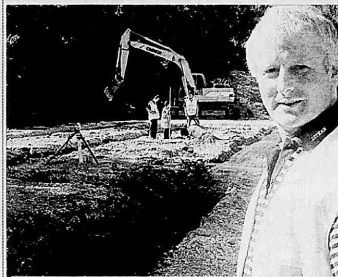
Inspecting the Foundations! Cork builder, John Browne, inspects the foundations being dug for the new homes earlier this week. Photo: Pat Kiely
