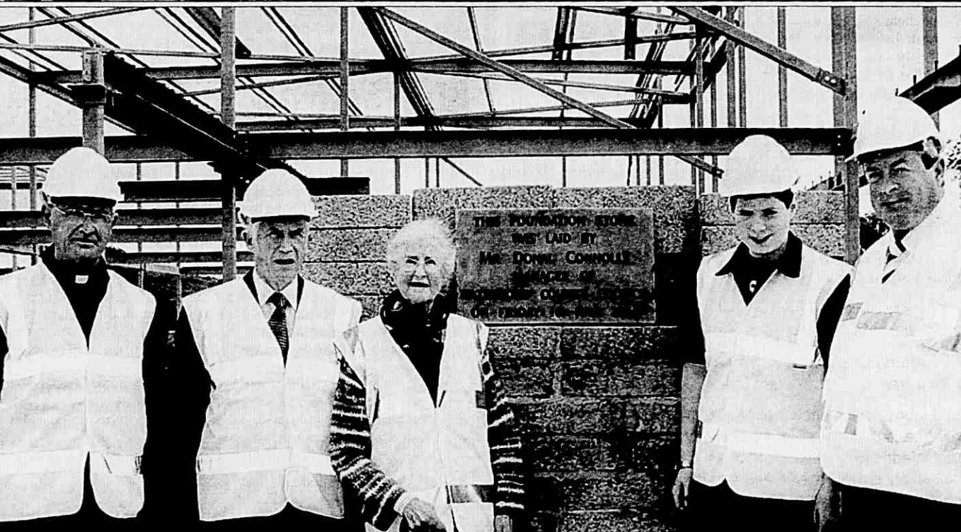
Laying of the Foundation Stone at the development of The Golden Meadows Retirement Village at the Burgery, Dungarvan were (left to right): Colin Fives, Donal Connolly, Co. Manager, Maureen Fives, (mother of the land owner), Daniel Lordan and Danny Lordan, M.D. Golden Meadows Retirement Villages. —(Photo: Sean Byrne).
