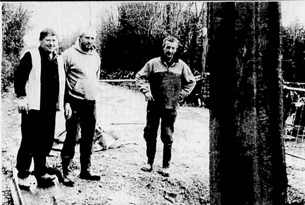
Left to Right" John Keating, Norman O'Neill and Richard Molloy at work on the public sewer in the roadway from Strandside North to Pinewood and as far as Knockateemore. The road is closed to facilitate the improvements. An alternative route is available via the N25 to Tarr's Bridge and along the N72 to Ballycoe Cross.
