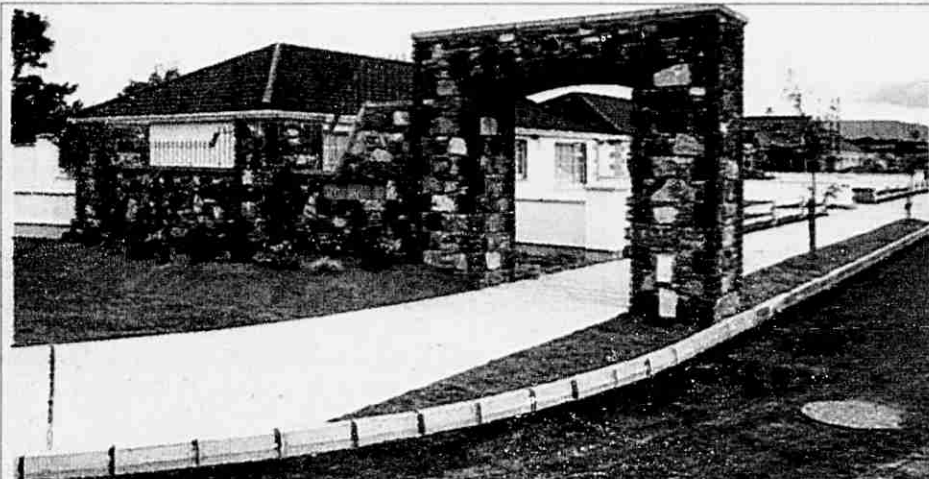
Construction of new homes at The Comeraghs, Stradbally is progressing well (see above) with particular emphasis on quality of work and finish. There is an increased interest in Stradbally due to its selection as Ireland's entry in this year's Entente Florale.
