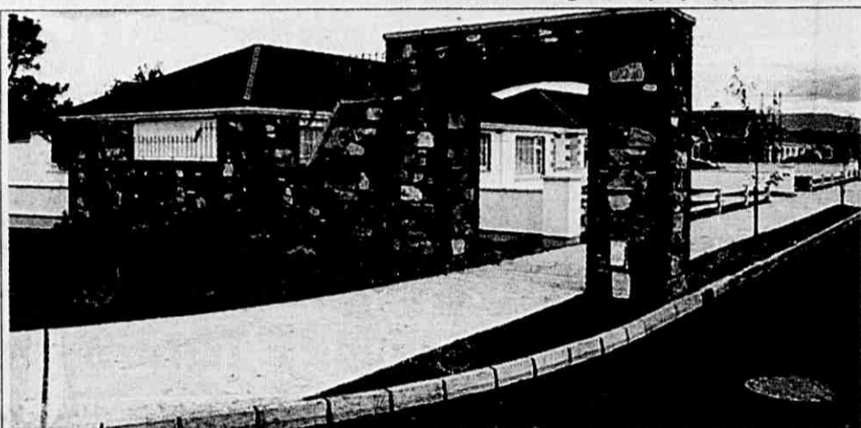
Construction of new homes at The Comeraghs, Stradbally is progressing well (see above) with particular emphasis on quality of work and finish. There is an increased interest in Stradbally due to its selection as Ireland's entry in this year's Entente Florale.
