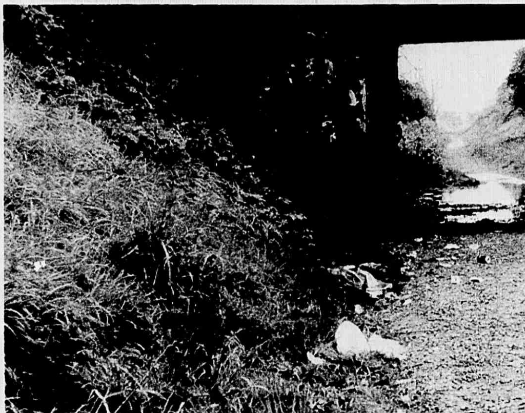
LITTER PROBLEMS — The above photograph shows the extent of the continuing litter problem beneath the bridge connecting the New Line and Murphy Place.
