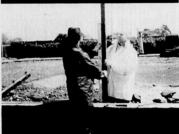
Work is in progress on the new tennis courts in Walton Park, Abbeyside.
