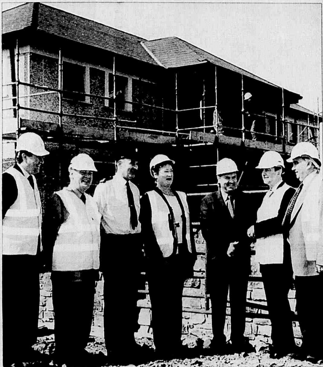
Pictured during the visit to the new Kilmacthomas Garda Station were (left to right) John Noonan, Flahavans Ltd., Cllr; Pat Daly, Chief Superintendent John Howard, Una Redmond, Project Manager OPW, Maurice Kirwan, Builder, Minister Martin Cullen T.D. and Cllr. Pat Leahy. —(Photo: Sean Byrne).
