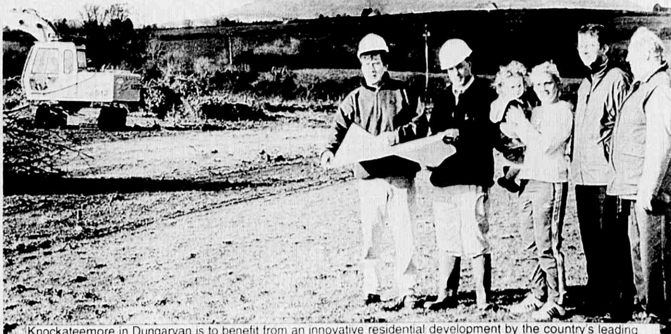
Knockateemore in Dungarvan is to benefit from an innovative residential development by the country's leading firm of home builders, McInerney Construction Ltd.
