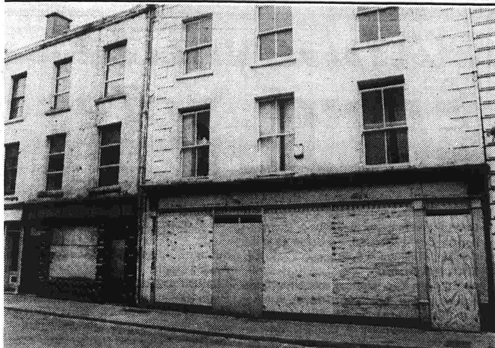
The derelict side by side buildings of the former Mulcahy's and Doocey's premises in Main Street, Dungarvan which are earmarked for a multi million pound development.
