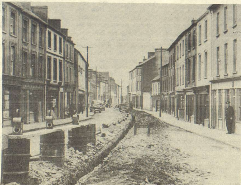
Down the road, workmen were putting down a new sewerage scheme and people generally were feeling the greatness of the inconveniences.
