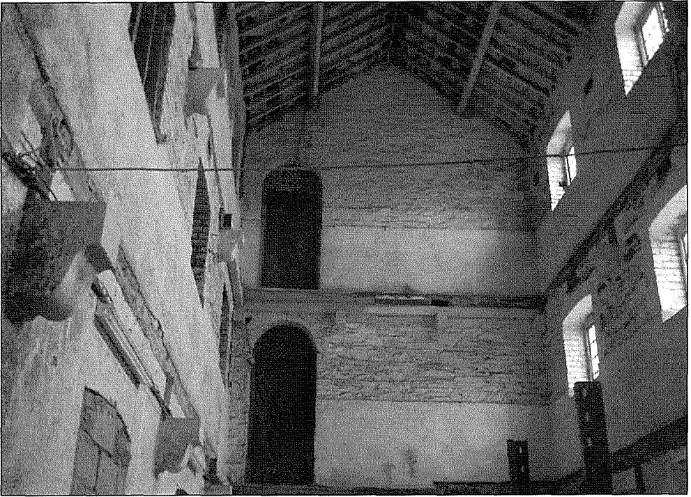
Plate 3: Internal view of the male dormitory. The mullions are clearly visible on the left hand side which held up the supports for the floors.
